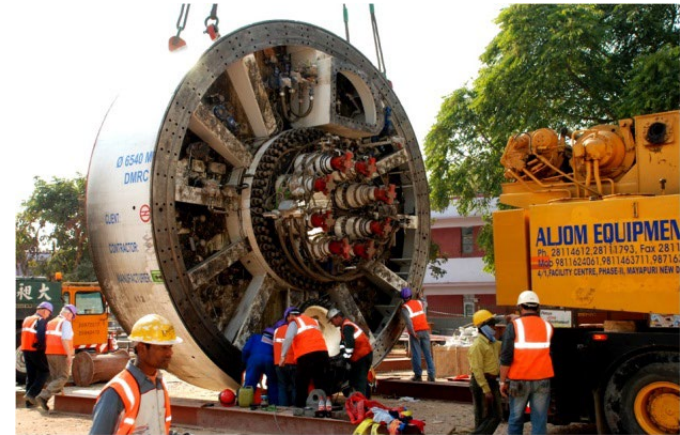
Assembling of a tunnel boring machine in Delhi Mass Rapid Transport System Project
